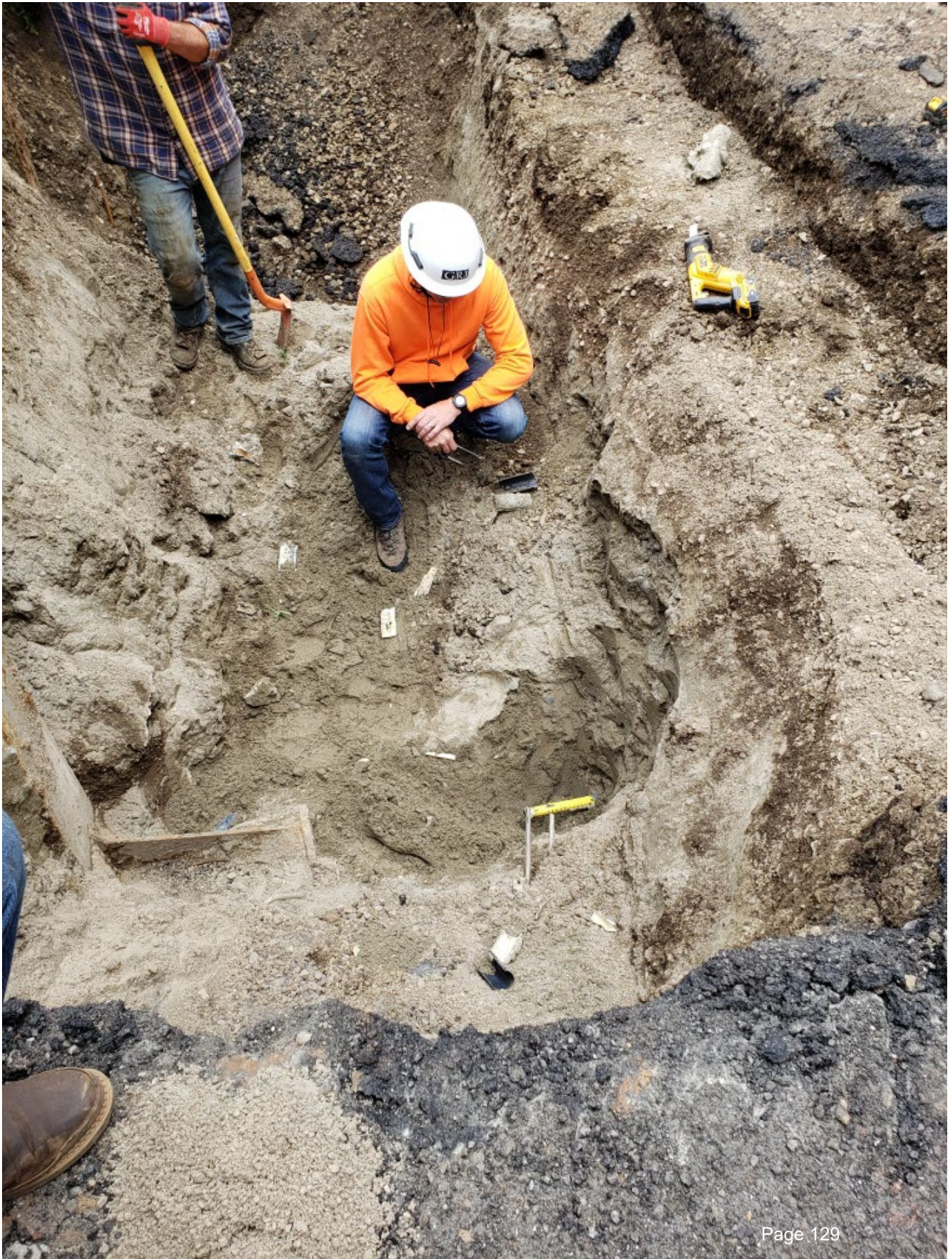
1: The end of the tieback here is bright yellow. It should be mounted to the flange on the left, but it has parted and moved back 36"
