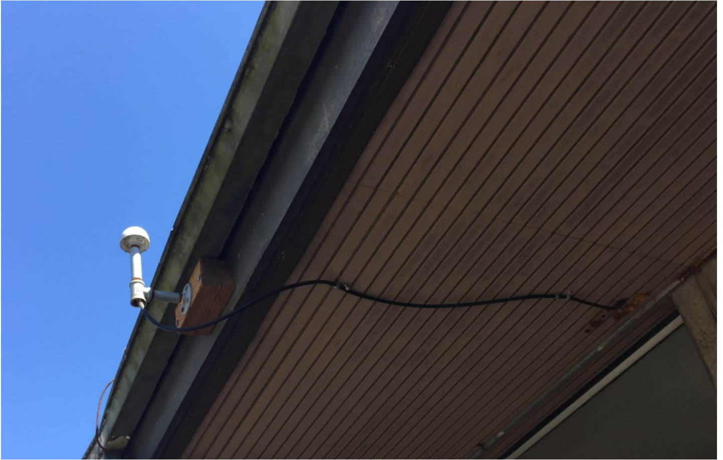
Figure 7 – Outdoor mounted GPS antenna resides on the frame of the roof.
