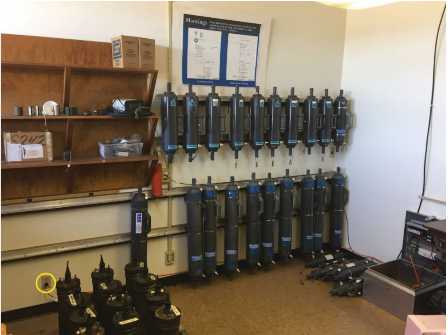
Figure 6 – The seismic station is powered by plugging into a nearby outlet (yellow circle). The black cord running up the wall to the ceiling from the enclosure connects to the outdoor mounted GPS antenna.
