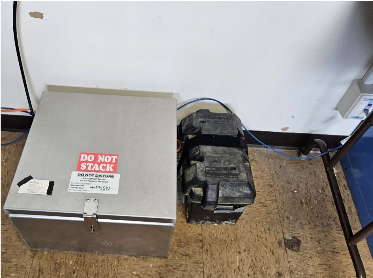
Figure 5 – Aluminum enclosure housing the 3-channel seismic sensor. The backup battery resides directly next to the enclosure. The station plugs directly into a nearby ethernet port for on-site internet.
