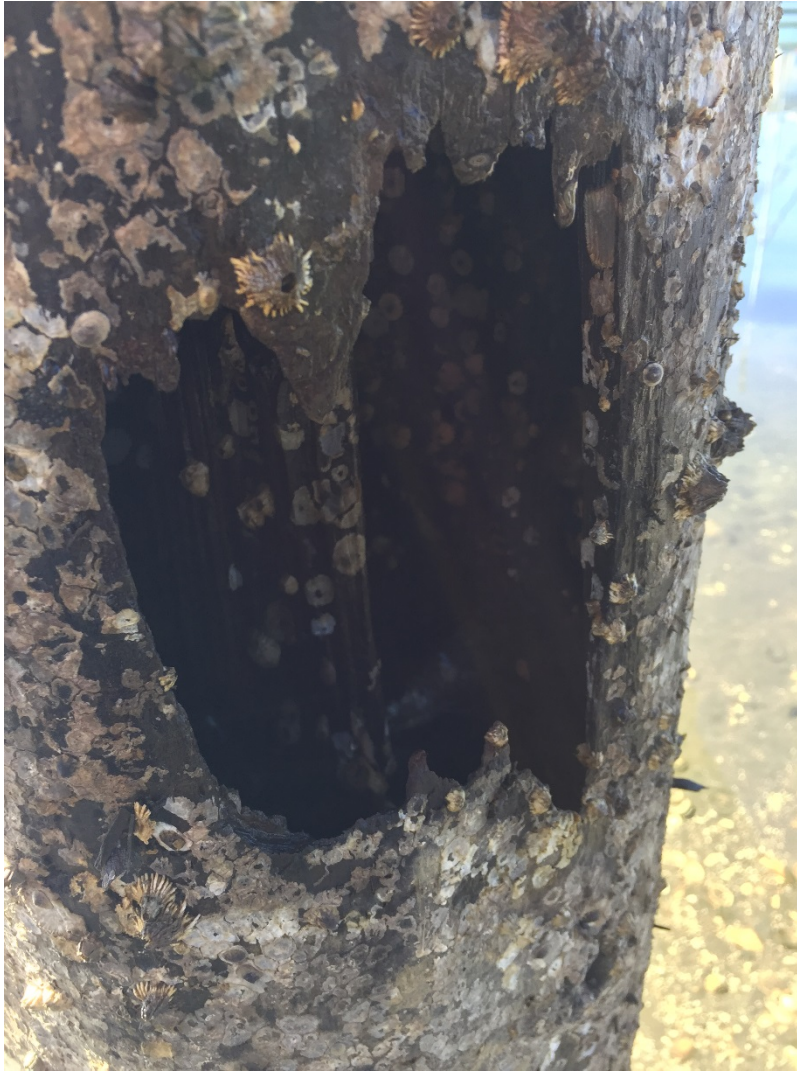
Figure 3. A piling on the Port Dock 5 pier with gaping holes above the mudline
