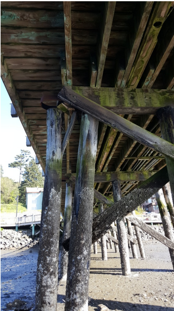
Figure 1. The top of a piling supporting the Port Dock 5 pier that has pulled away from its placement.
