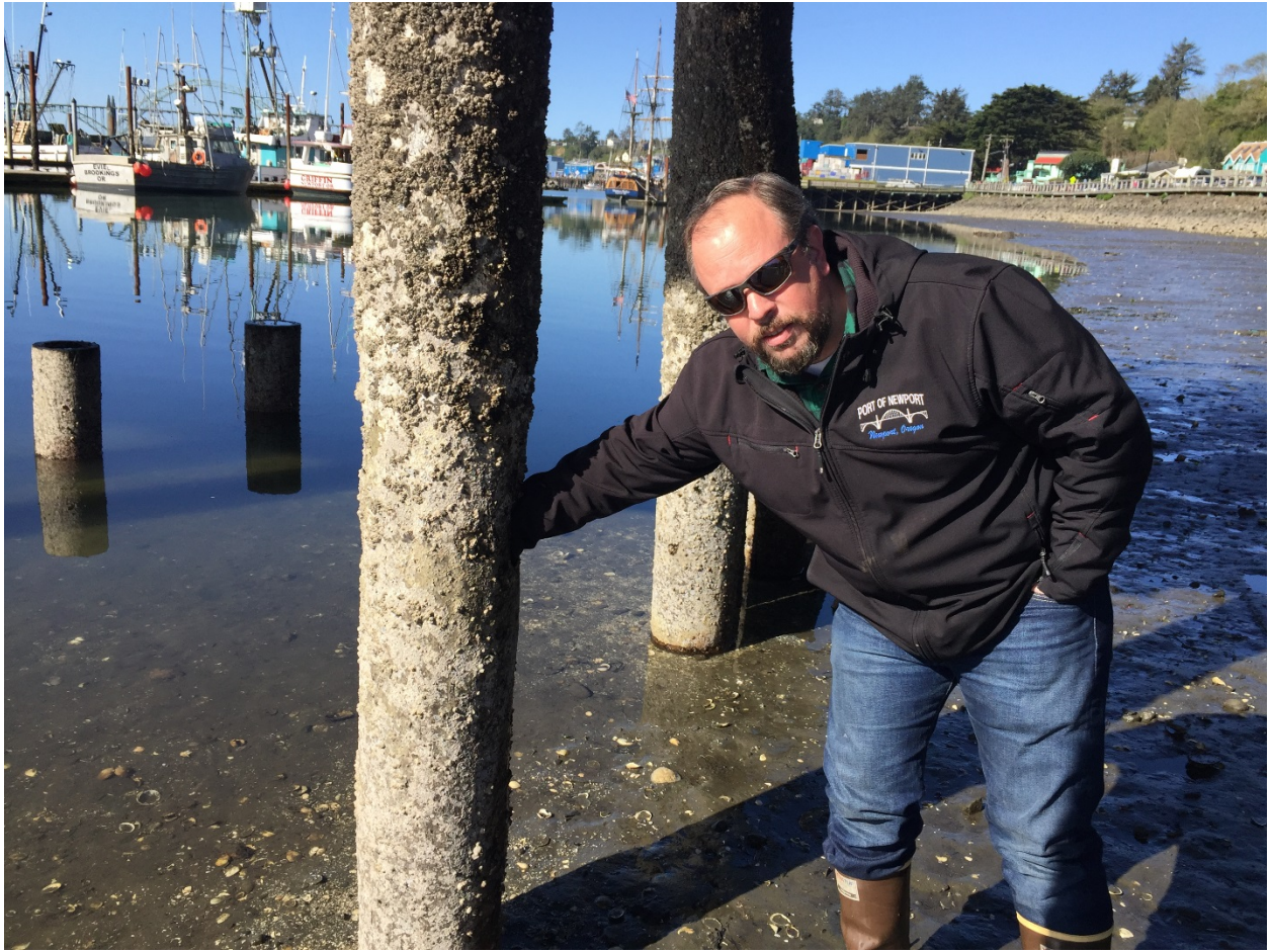
Figure 1: The Port's Director of Operations, Aaron Bretz places his hand inside a hole in a piling supporting the Port Dock 5 pier structure.
