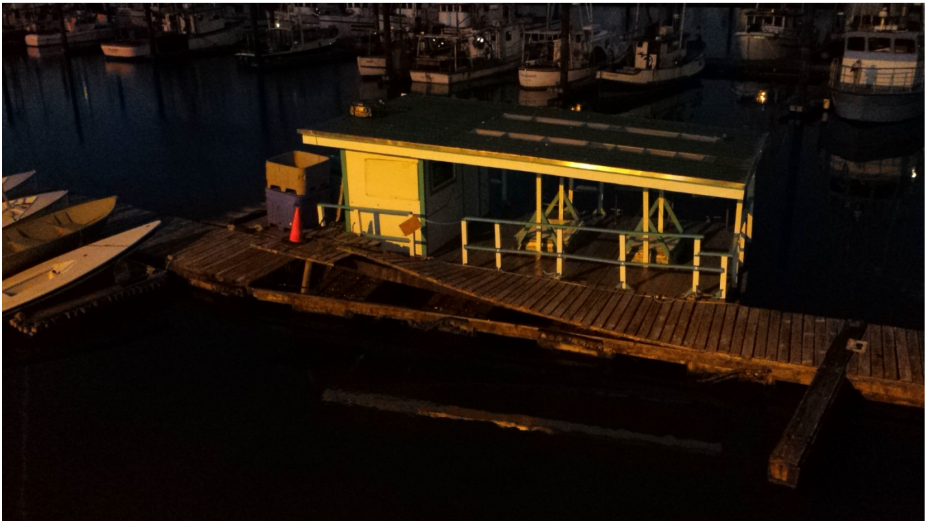
Figure 3: Damage to Dock 7B from a broken piling
