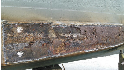
Figure 2 Excessive pitting and rust, doubler plate
