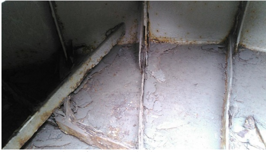
Figure 1 Failing frames in the lazarette
