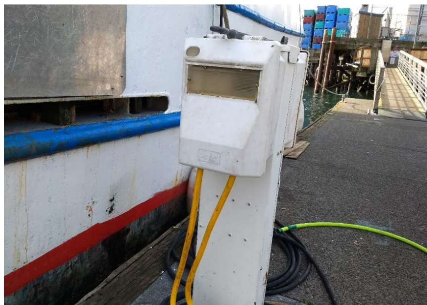
Photo 4 – Port Dock 3 – Electrical Pedestal
