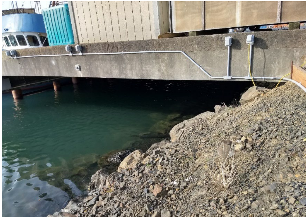
Photo 15 – Hoist Dock – Electrical in Tidal Zone
