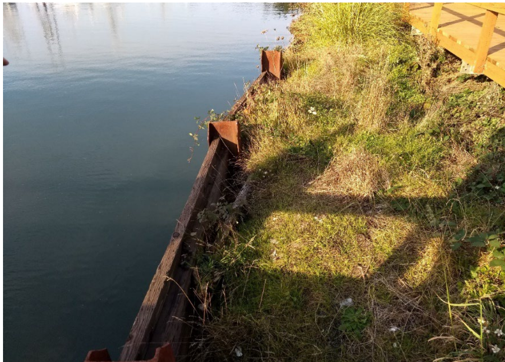
Photo 9 – Port Dock 7 – Erosion
