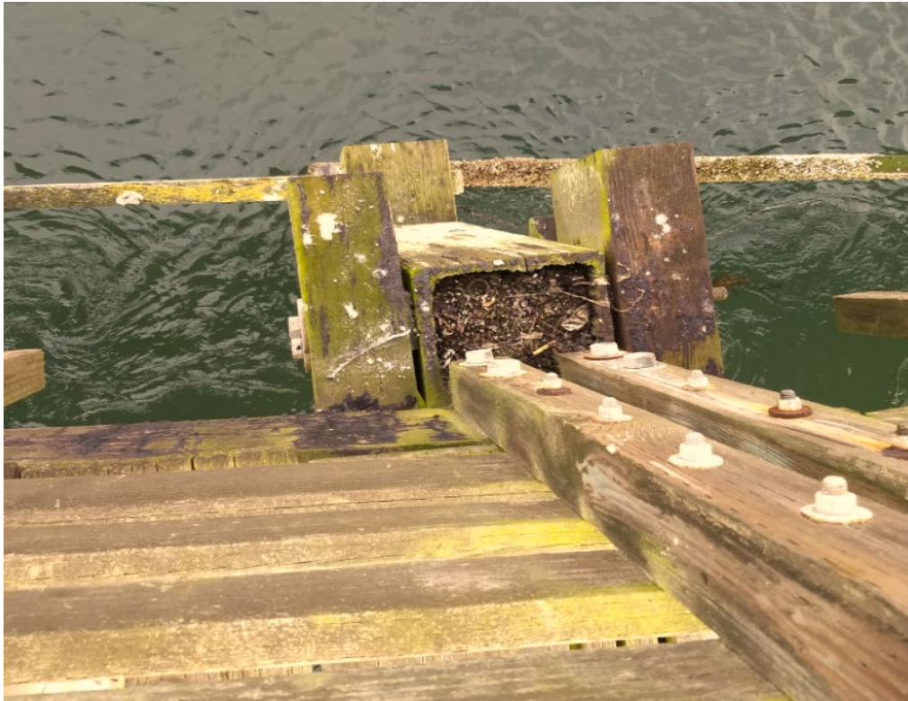
Photo 26 – Fishing Pier – Railing Support
