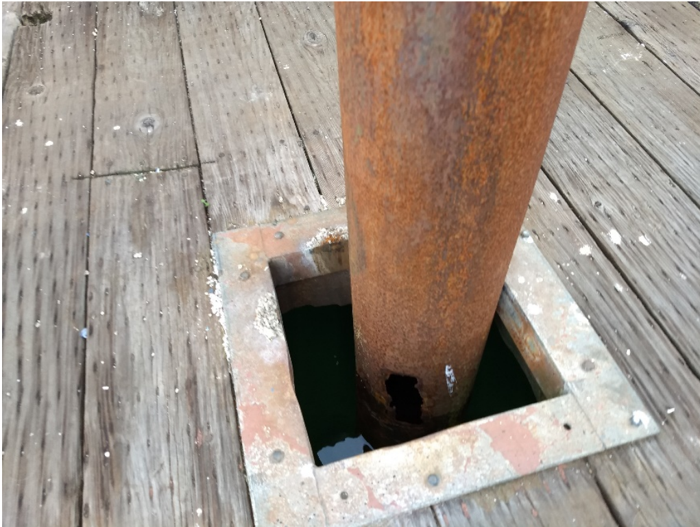
Photo 18 – Swede’s Dock – Damaged Pile
