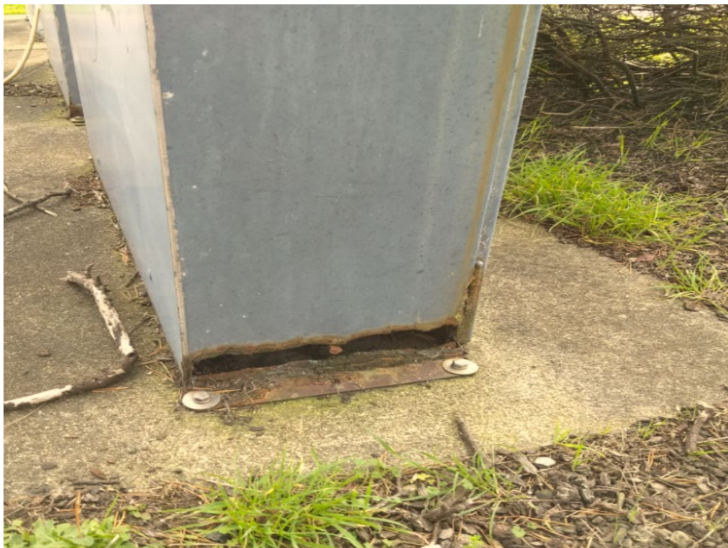
Photo 29 – South Beach Marina – Load Center Base Corrosion
