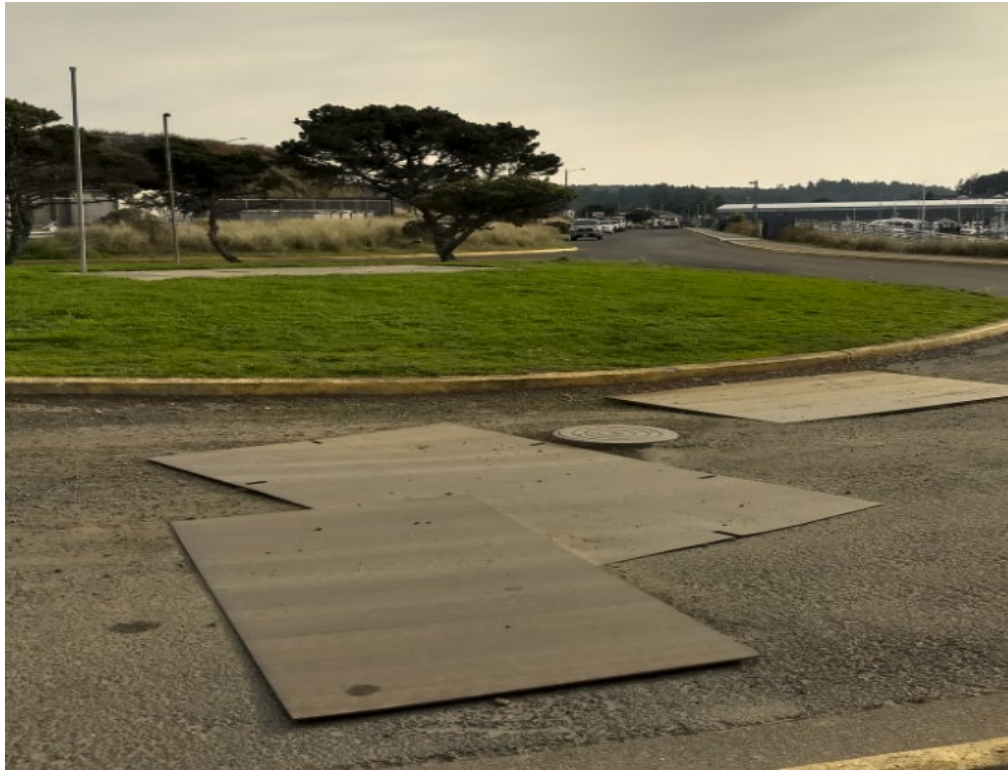
Photo 32 – Patched Road near Fuel Dock
