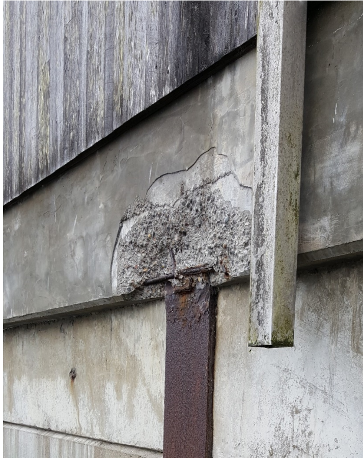
Figure 9. Concrete Spalling at Pile Cap
