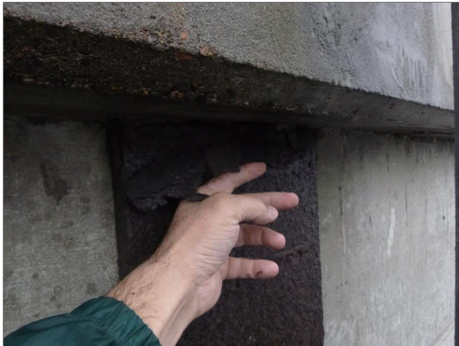
1(d). Typical chloride induced corrosion damage under the pile cap (8 October 2018)
