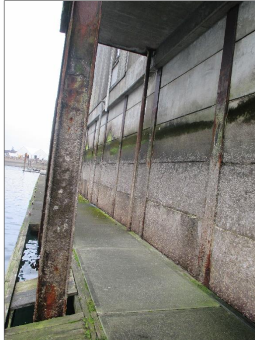
Figure 2. Concrete lagging existing conditions (There are surface effects from water; however, the overall visual inspection seemed acceptable at this point.)
