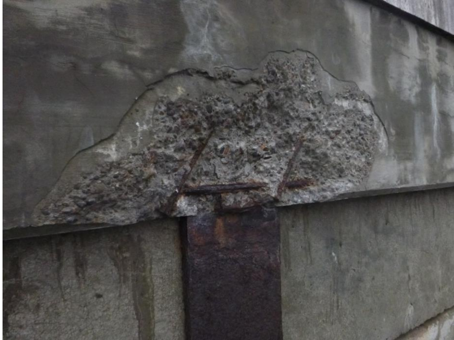
3(a). Concrete spalling on pile cap (Pile No. 42, see as-built drawings)
