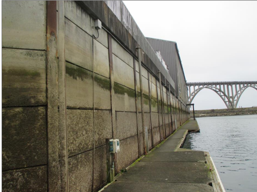
1(a). Corrosion on soldier piles (27 February 2018)
