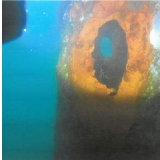
Photo 10: Corroded pile near slip 25
