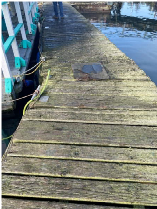
Photo 3: Hole with decayed patch in Dock B
