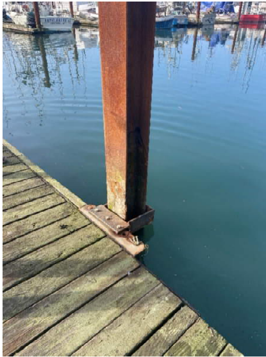
Photo 14: H Pile on Dock X near the gangway. Note heavy corrosion near the waterline.
