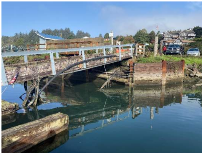
Photo 19: Fallen utilities on gangway. Also note missing lagging in wall.
