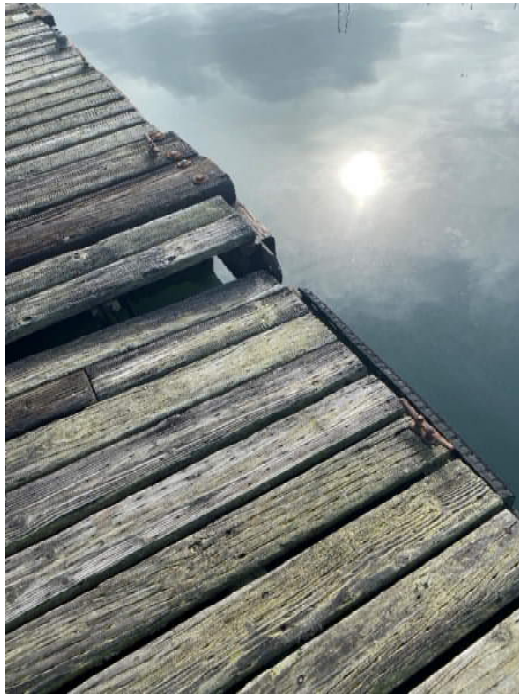
Photo 2: Missing hardware near space 15 on Dock B
