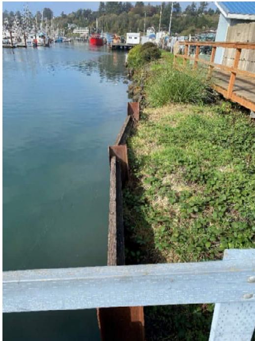
Photo 18: Leaning bulkhead wall
