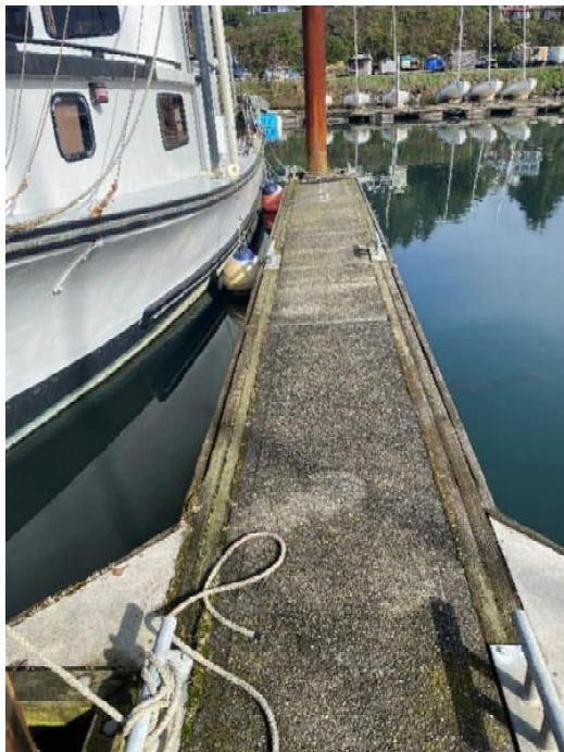
Photo 9: Concrete finger, showing a lean to one side
