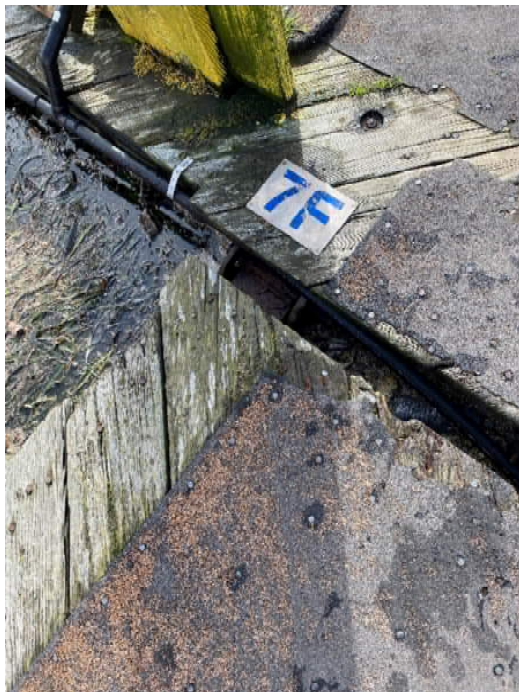
Photo 17: Missing hardware at intersection of Dock X and Dock E/F
