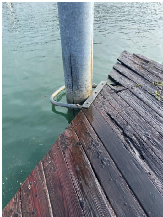
Photo 13: Typical pile hoop attachment
