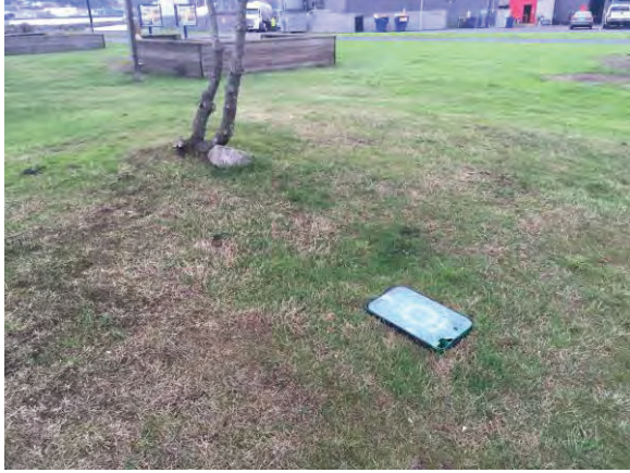
Picture #19. Utility box
