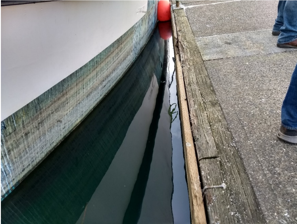
Photo 5 – Port Dock 3 – Timber Rub Rail/Wale Damage
