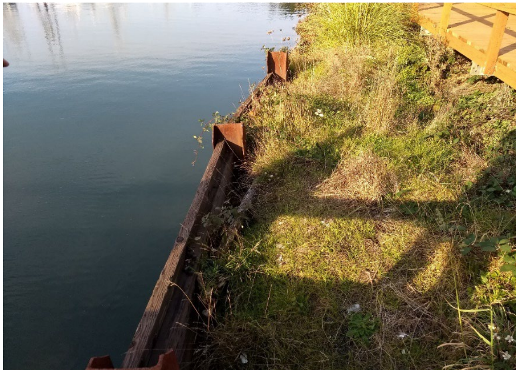
Photo 9 – Port Dock 7 – Erosion
