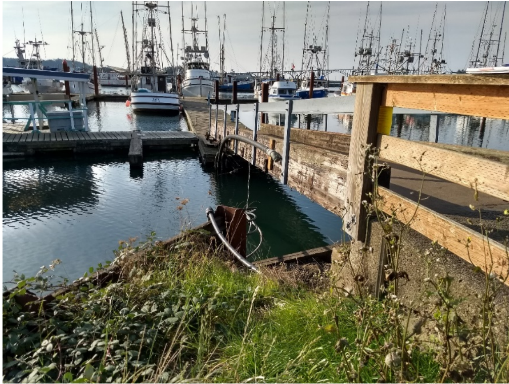
Photo 10 – Port Dock 7 – Approach
