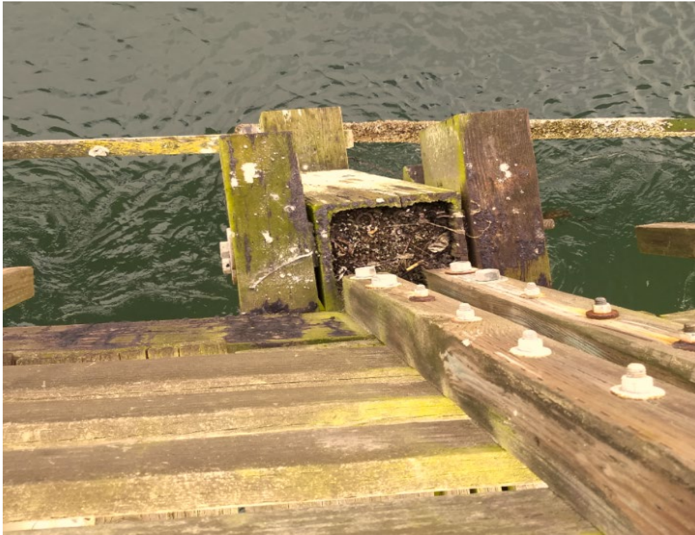
Photo 26 – Fishing Pier – Railing Support
