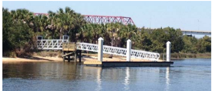
HDR provided design, permitting, and construction services for a new 60-foot by 8-foot floating dock and associated access on Exchange Island near downtown Jacksonville, Florida.
